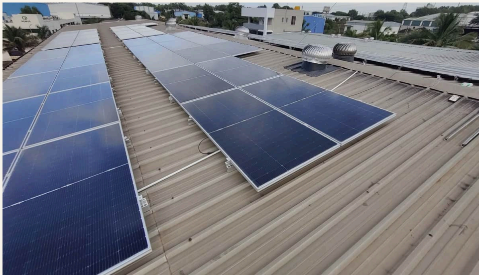
Rooftop solar On the production shed at Belur.
